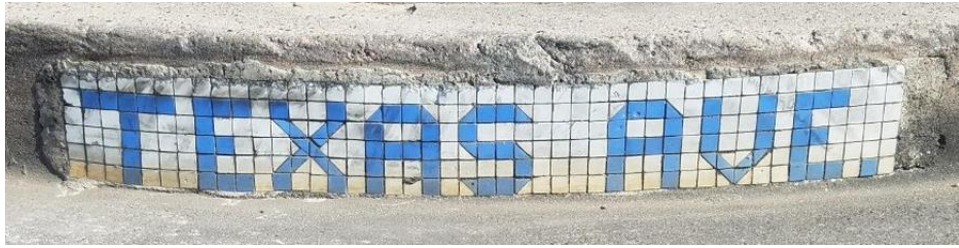
Image 16. This is the only intact Texas Avenue marker and one of only a handful of markers remaining from the 1930 curb and gutter project. It is located at N. First Street.
