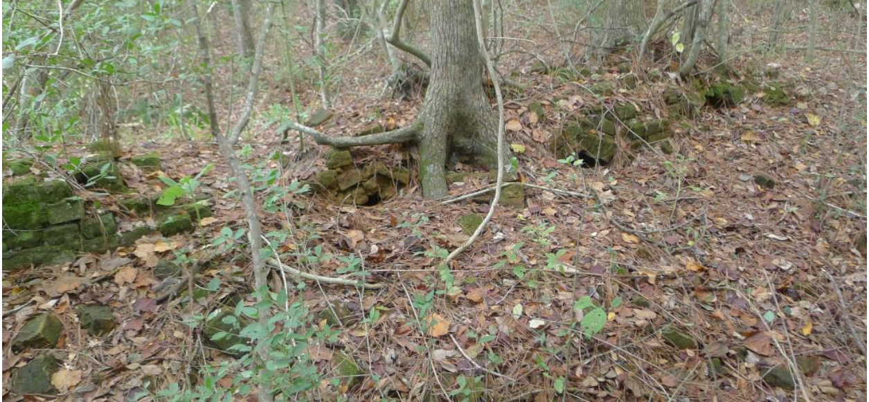
Image 13. Three eyes in this Cedar Bayou kiln are barely visible in this photograph. Almost the entire kiln has been covered by alluvium from more than a century's worth of floods. Image by author.
