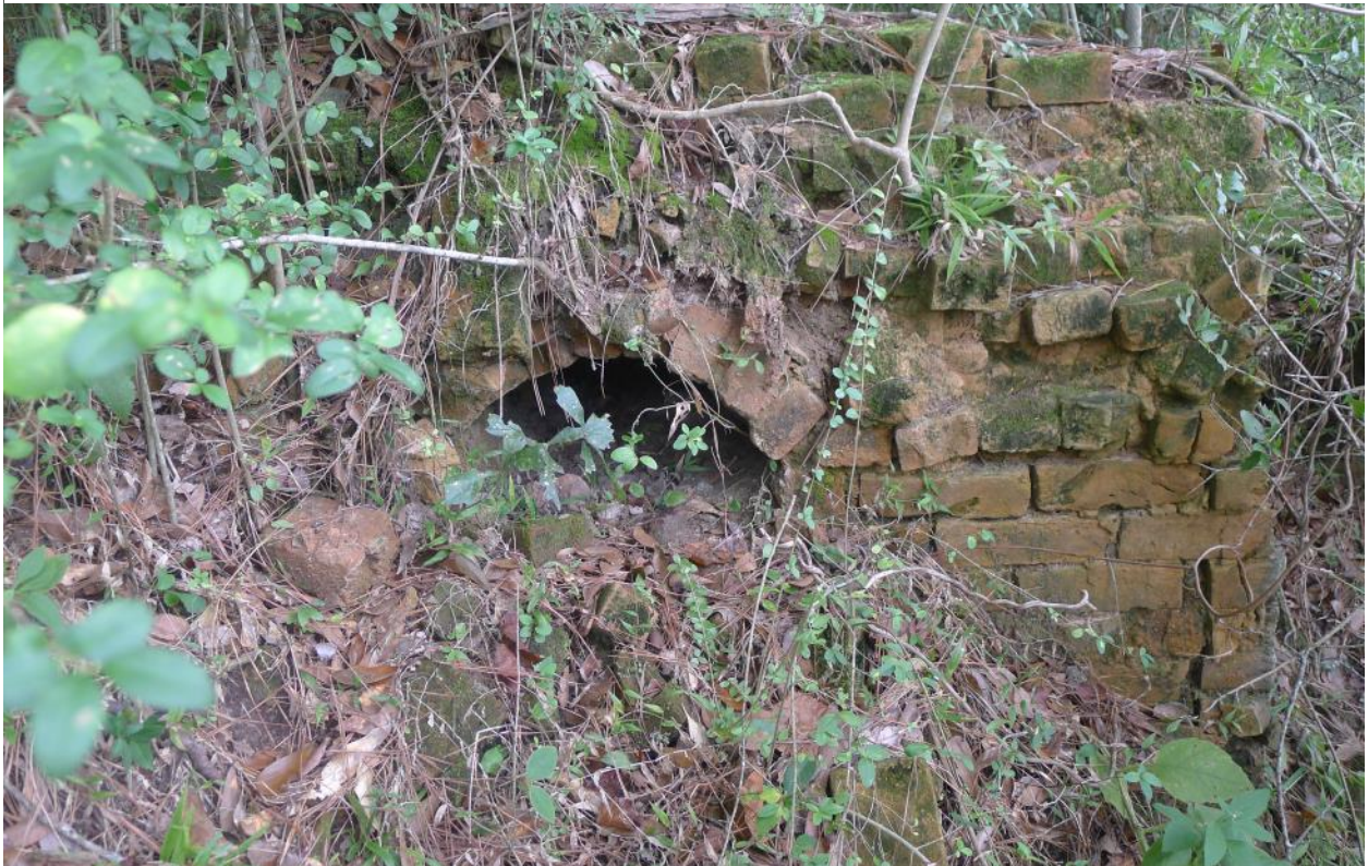
Image 14. The corner of the kiln closest to the water's edge has more of the kiln visible due to the silt washing over the edge of the bank. The eyes of the kiln have been filled and almost the entire kiln has been covered with silt. Compare the construction of the eye with the Williamsburg kiln above. Image by author.
